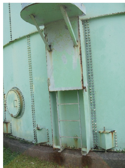
Fig.1c: Deteriorating condition of Upper Amouli Tank.
