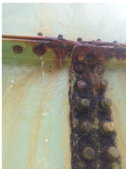
Fig.1a: High leakage from rusted panels and bolts.
