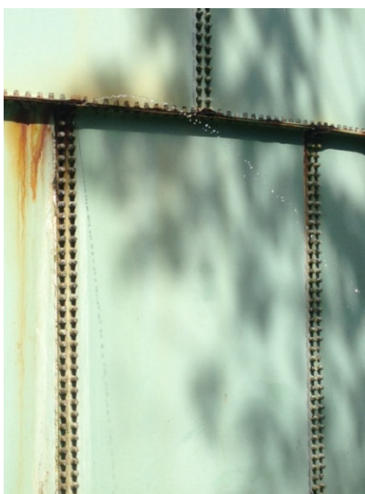
Fig.1b: Water spraying out from rusted tank panels.
